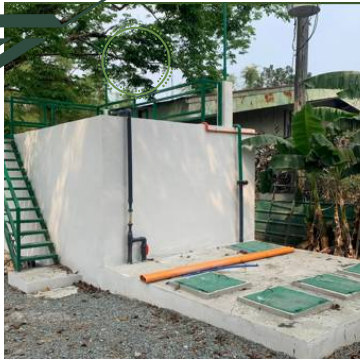
50 CMD SEWAGE TREATMENT PLANT
