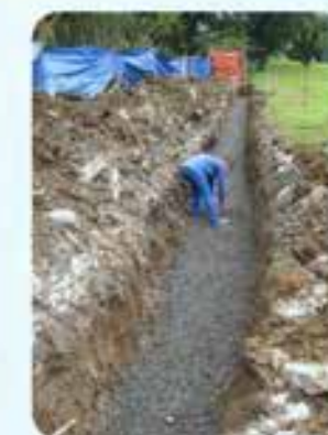
CHB fence at Hole # 3 NC Before
